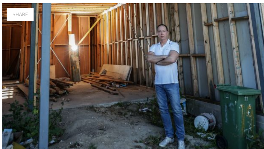
Tony Veleski in front of the two Footscray townhouses that will be so badly built they will have to be demolished. Photo: Jason South
